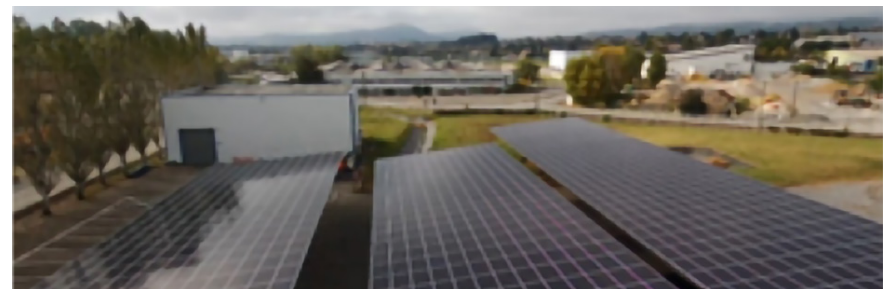
Solar power installation at Bausch + Lomb Pharmaceutical site in Aubenas, France.
