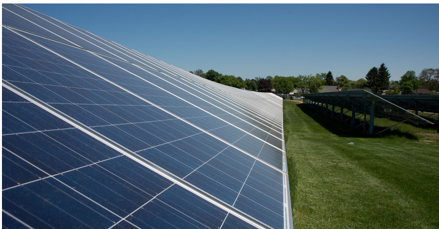
The solar array at the Rochester, NY, United States Optics Center.
